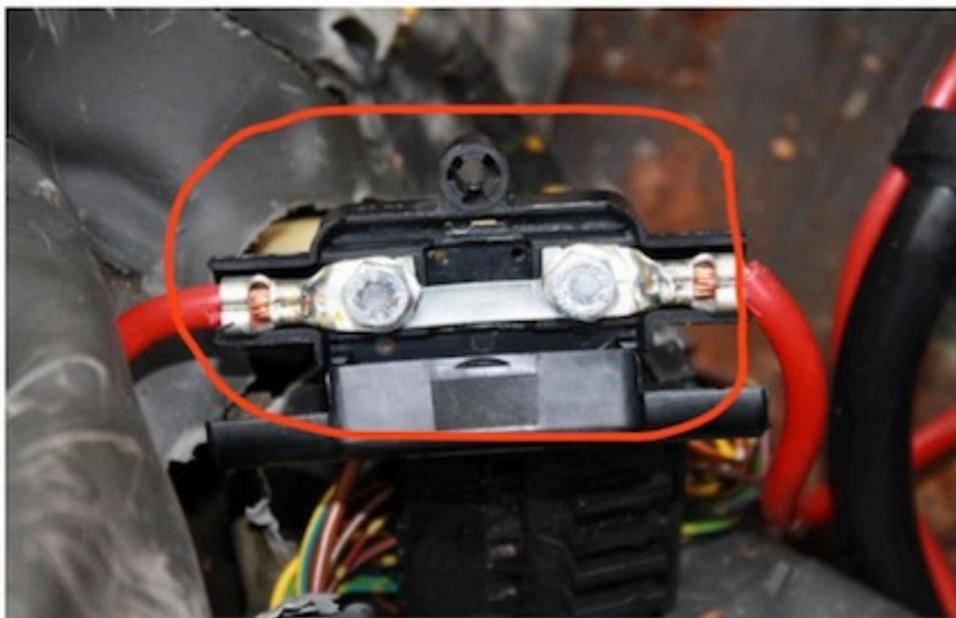
Fusible Link B with cover open.
